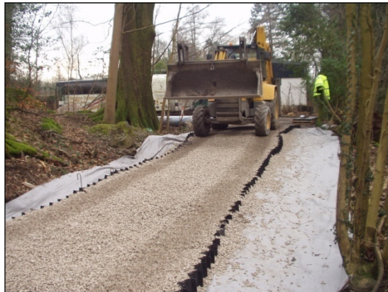
Photo 4- once filled the system can support plant to carry aggregate to the fill area
